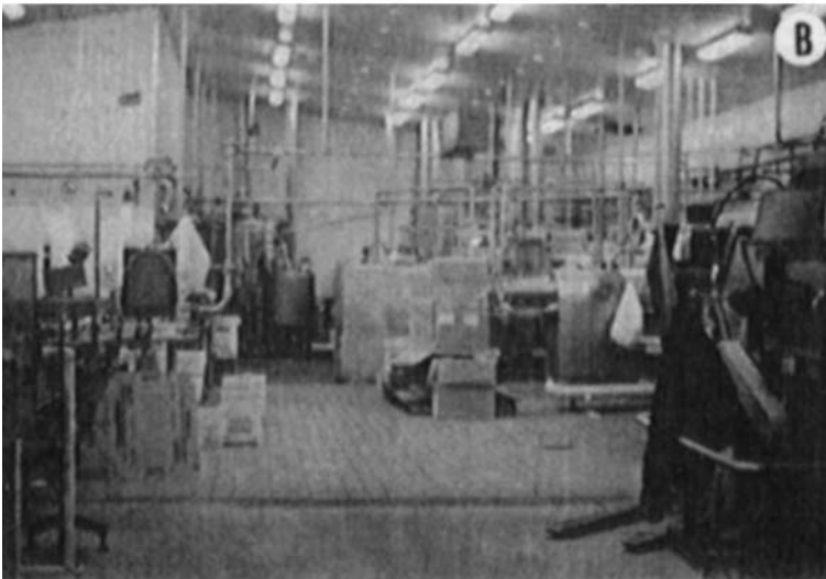
Figure 19 Oil processing facilities. (A) Oil deodorizer and (B) margarine packaging plant in Melbourne, Australia.
